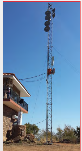
Wi-Fi Receiver Station and Control Room
