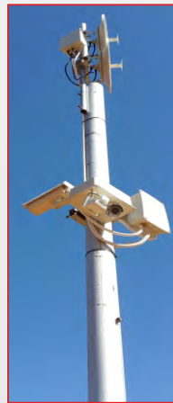
Wi-Fi Transmitter Station
